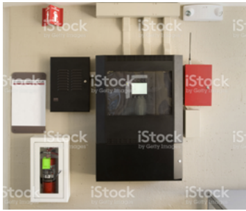
Security and fire alarm
