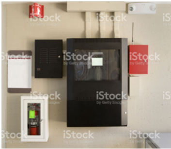
Security and fire alarm
