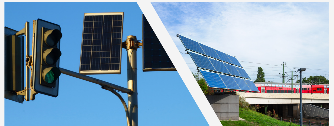
Traffic signal systems
