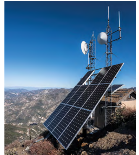
Remote Telecom Stations
