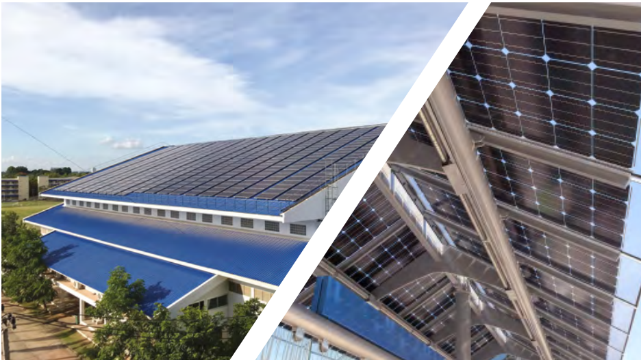
Residential Installations, Off-Grid Power Systems
