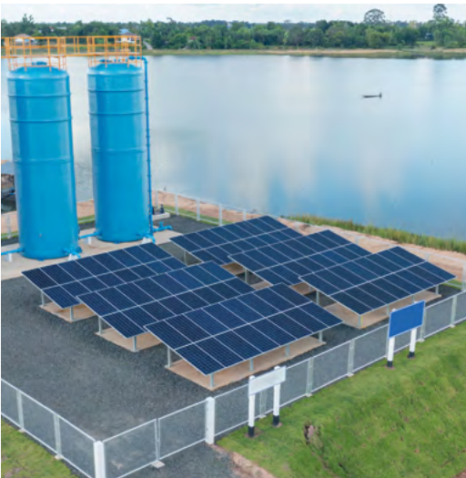
Water Pumping Systems
